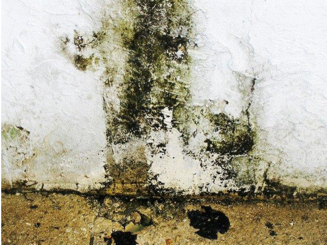
Figure 01: Black Mold Spread on Walls
